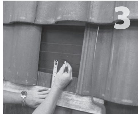
3 Use a straight edge and measure up 6 5/8" from bottom of tiles to center of the mount over the center of rafter.
