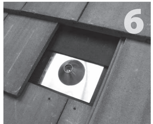
6 Take care to do a quality installation. When using the paper method, cut a piece of paper 18" wide to slide under the course above, and over the primary flashing of the mount. See reverse side for details on the three-course method.
